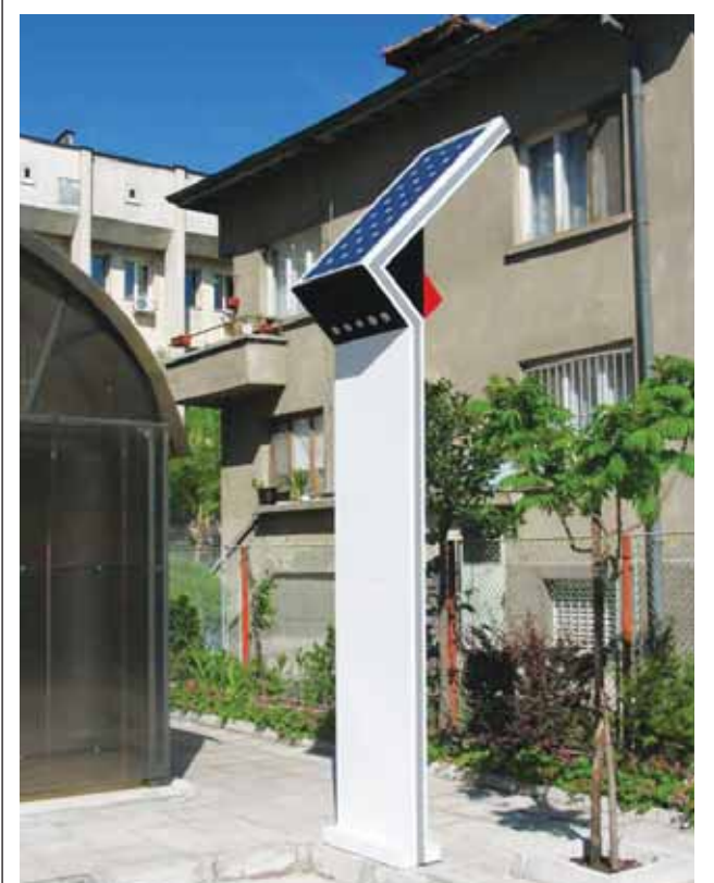
The lamps work on photovoltaic principle as supply is from a storage battery
